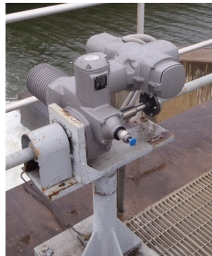
Figure 4 - Electric motor installed on one of the gates of the Rice Lake dam
